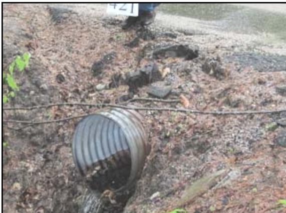
Above photo depicts an unstable culvert outlet in which road shoulder sediment is washing into a stream leading to Moose Pond.
